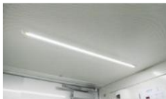
Ceiling LED lighting
